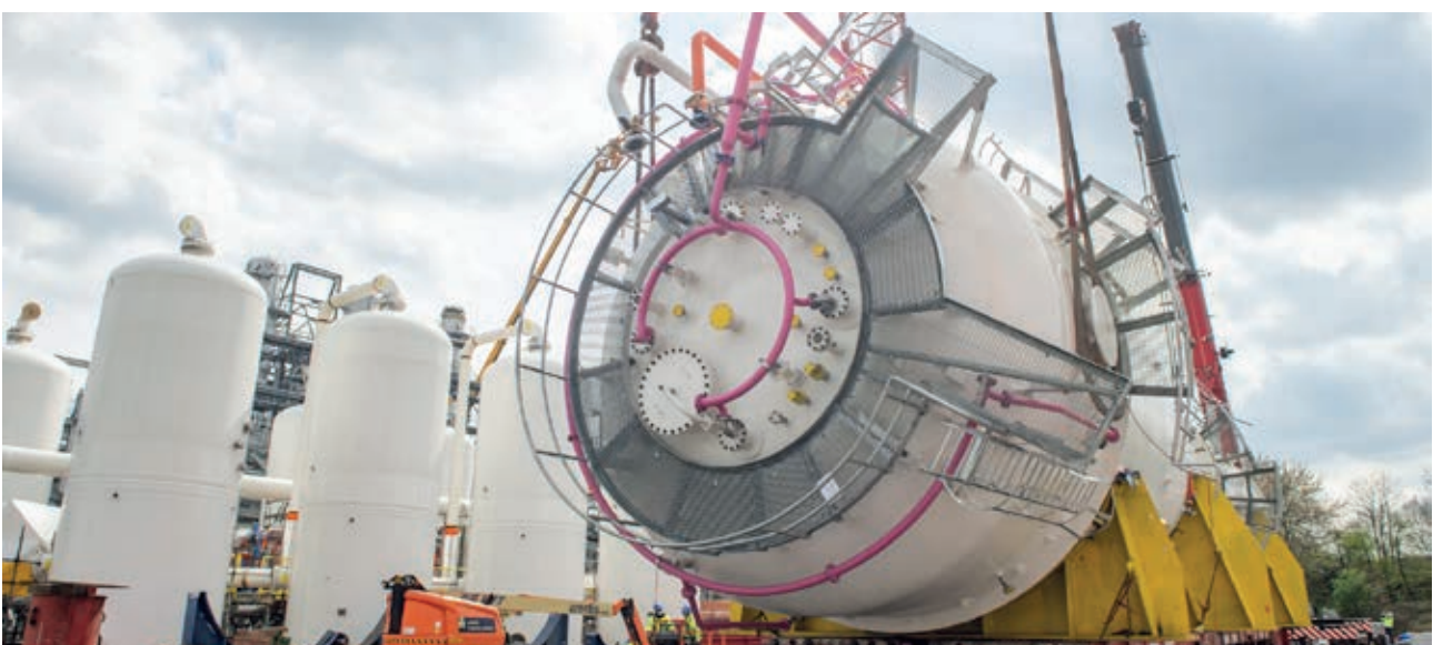
Hoisting of bioreactors for carbon-neutral steel production in ArcelorMittal Belgium's Steelanol plant in Ghent.
